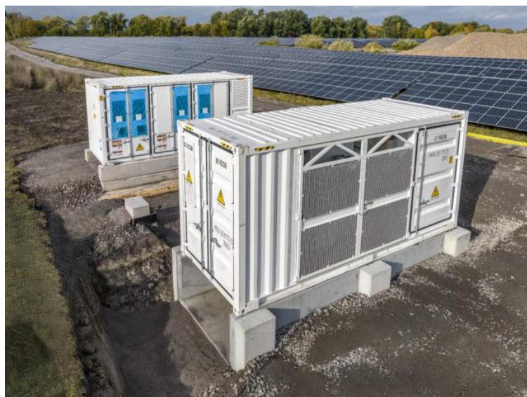
Figur 5. Huawei BESS 2MWh/2MW med Smart Transformer Station (STS) i Linköping.
